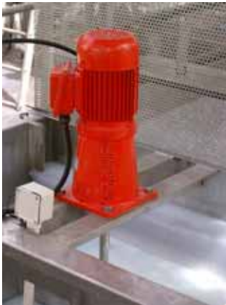
direct driven mixer on an open top tank
