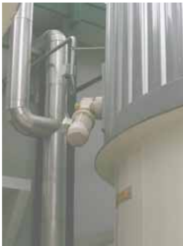
2.2kW side Entering Mixer 100,000 litre milk storage silos
