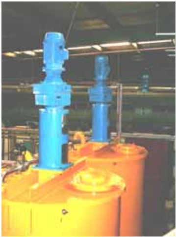
Series 75 mixers 15,000 litre slurry storage tanks
