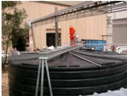
30,000 litre water treatment balance tank
